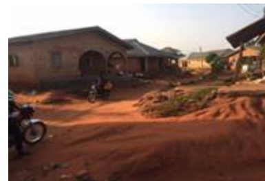
Plate 4: Effect of erosion on existing road
